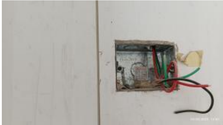
Electrical Switch Board
