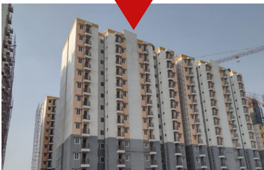
140 KW on-grid solar PV 39% of Roof Area covered by PV ACC blocks on roof
